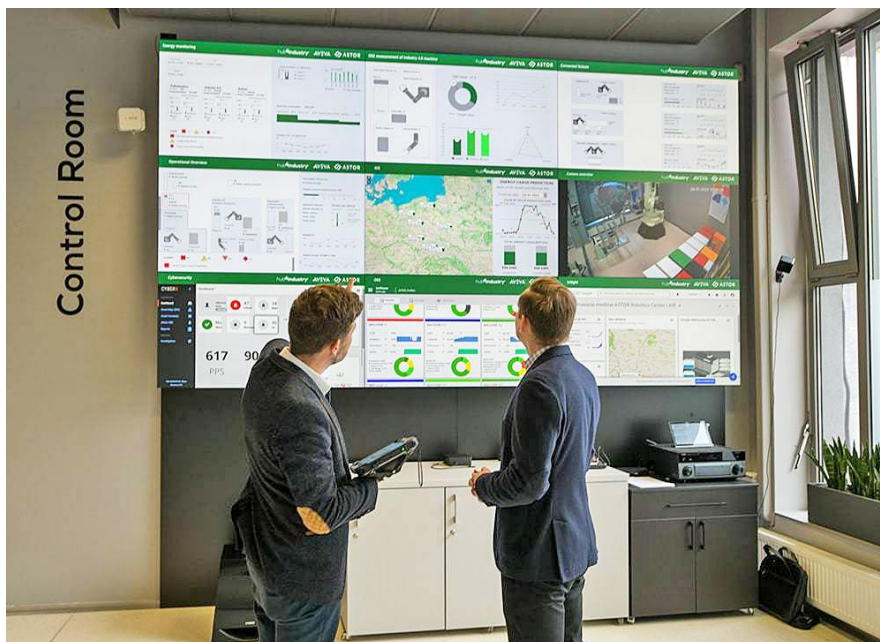
System klasy Control Room
