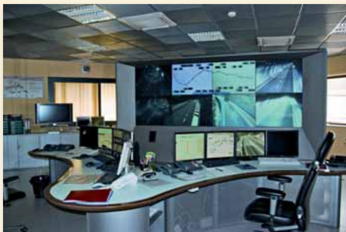
Figure 1: Central control headquarters A32 motorway.
